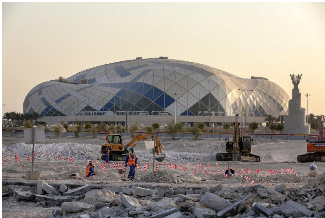
Workers seen at the construction site of Lusail Stadium, a venue for 2022 FIFA World Cup football matches. © Valery Sharifulin/TASS
